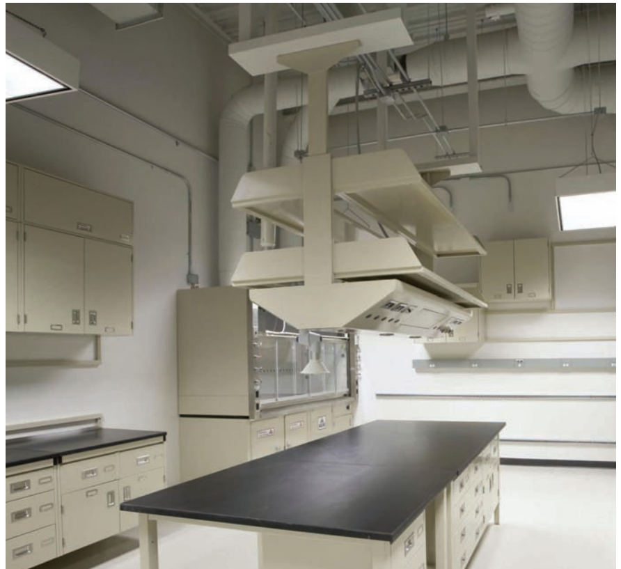
Chameleon™ service carriers can be suspended or flush mounted from the ceiling and are available in many configurations.
